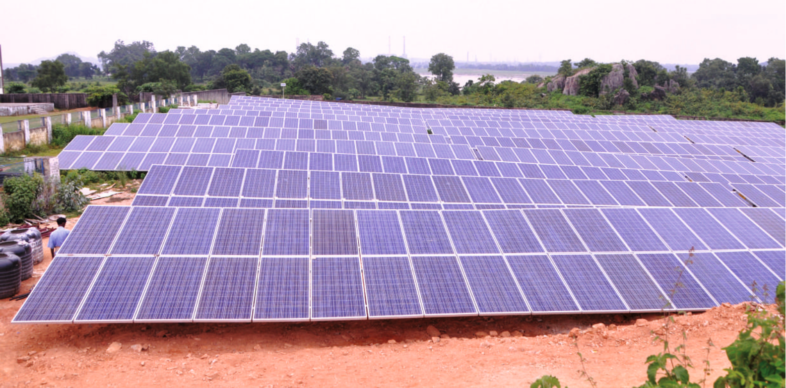
A solar power plant at Mahanadi Coalfields Limited in Sambalpur, Odisha
